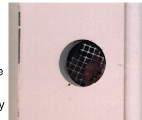
Screening attic vents is a way to prevent nesting.
